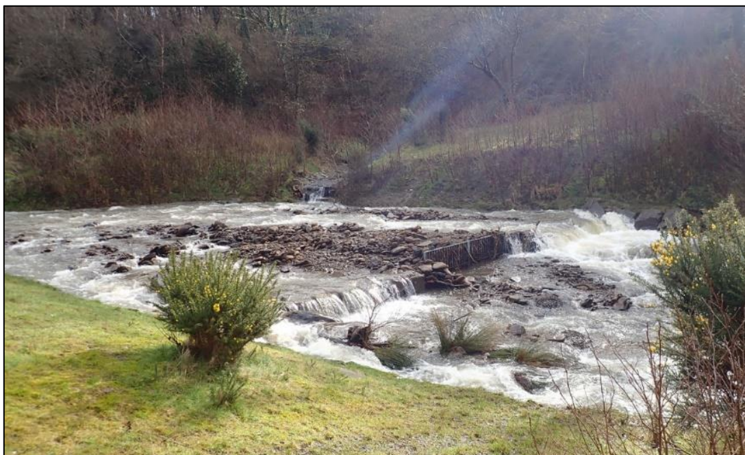
Figure 22: Initial upstream debris screen in the Nant Cae Dudwg watercourse (captured by RCT's Flood Risk Management team on 17 th February 2020)
