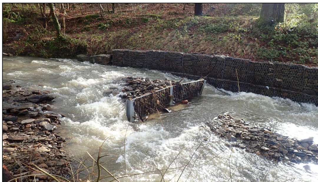
Figure 23: Second upstream debris screen in the Nant Cae Dudwg watercourse (captured by RCT's Flood Risk Management team on 17 th February 2020)
