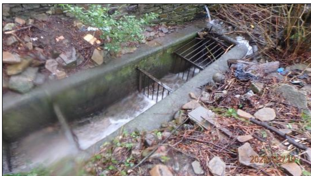
Figure 7: 'Culvert Inlet 3' to the rear of Dumfries Street which surcharged during Storm Dennis (captured by RCT's Flood Risk Management team on 19 th February 2021)
