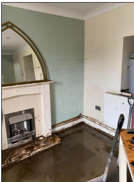
Figure 7: Water depth marks in a property at Cilfynydd Road following Storm Dennis (image provided by resident)
