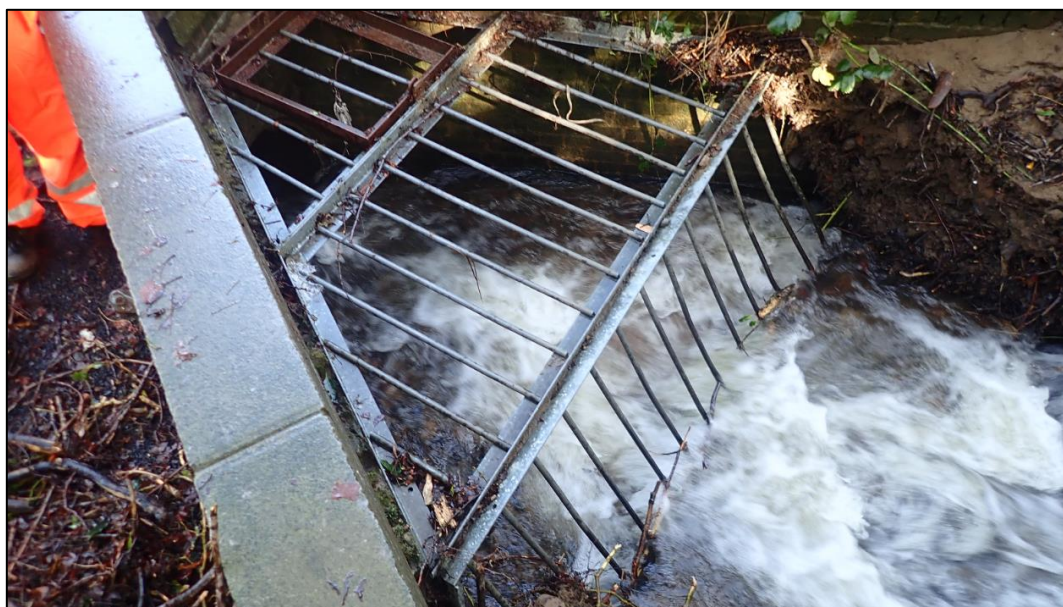
Figure 19: Ely Brook culvert inlet to the rear of Pontshonnorton Road which surcharged during Storm Dennis due to blockages at the inlet (captured by FRM officers on 17 th February 2020 following clearance works)
