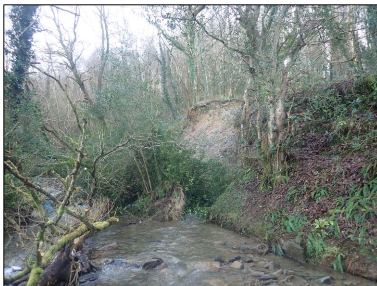
Figure 26: Photo of localised landslip on the embankment of the Nant Cae Dudwg watercourse (image captured by RCT's Flood Risk Management team on 02/03/2020)
