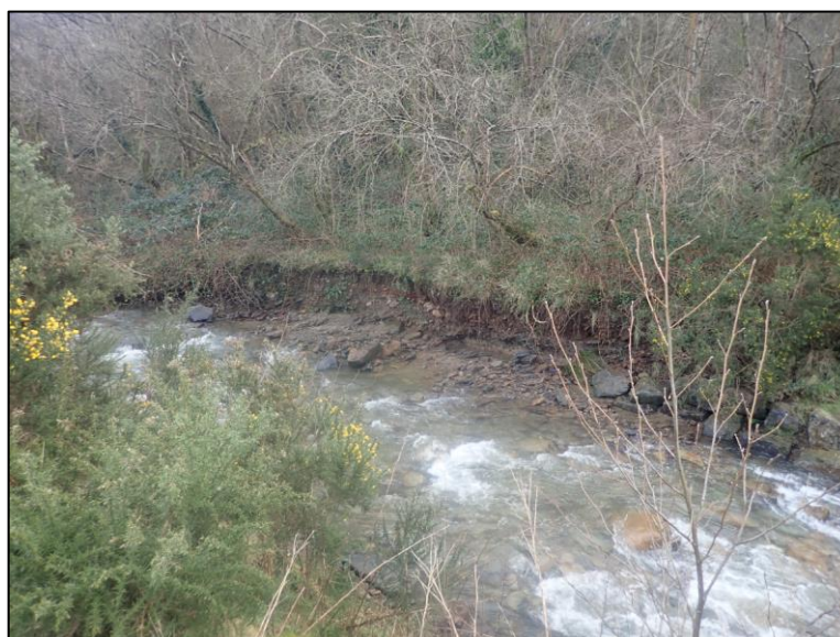
Figure 27: Photo of embankment scour to the Nant Cae Dudwg watercourse (image captured by RCT's Flood Risk Management team on 02/03/2020)
