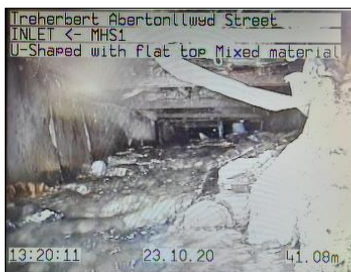
Figure 14: Internal view of 'Abertonllwyd Street Culvert Network 1' looking up towards 'Culvert Inlet 2' (CCTV survey footage captured 23/10/2020)
