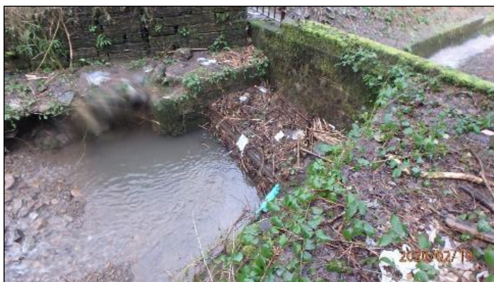
Figure 23: Photo of debris accumulation in the upper reaches of the Nant Coedcaetylefforest ordinary watercourse (below the A4061) (captured by RCT's Flood Risk Management team on 19/02/2020)
