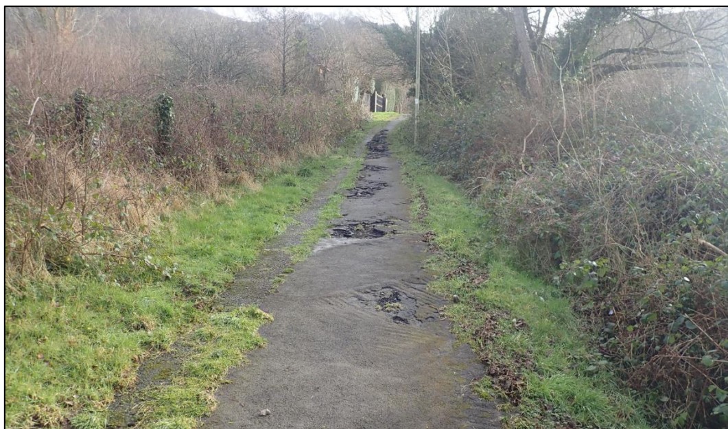
Figure 11: Evidence of damages to the top of the path looking up towards Heol Nant (captured by FRM officers on 17 th February 2020)
