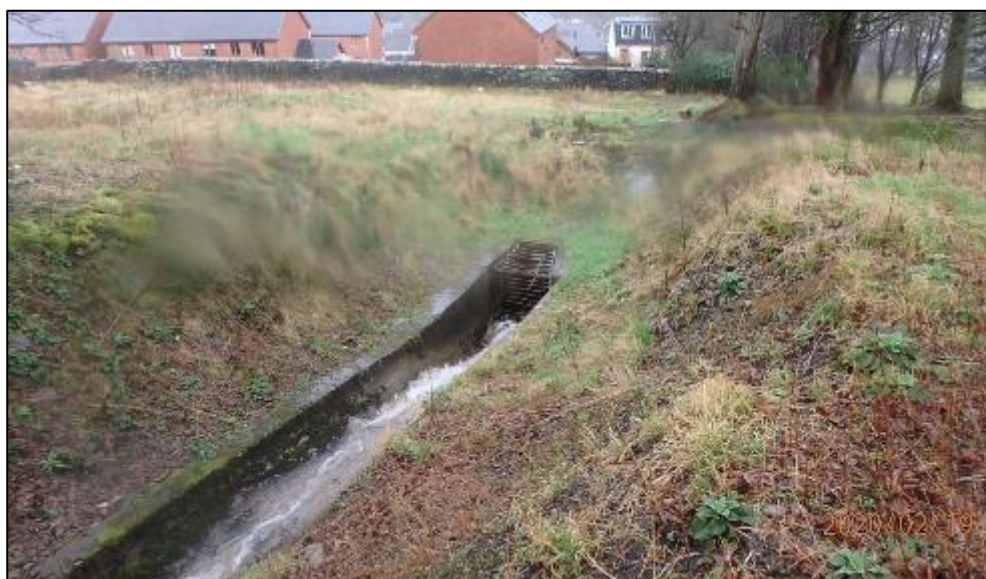
Figure 24: Culvert inlet at Area 2 which conveys the Nant Coedcaetylleforest ordinary watercourse towards Area 3 (captured by RCT's Flood Risk Management team on 19/02/2020)
