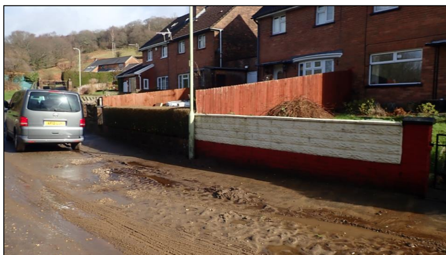
Figure 10: Road damages and debris deposited along Heol Cronfa following the storm event (captured by FRM officers on 17 th February 2020)
